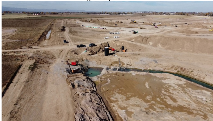
Prairie Song Pump House Location
