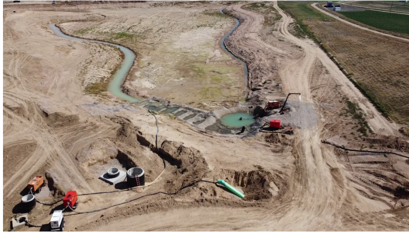
Prairie Song Pump House Location
