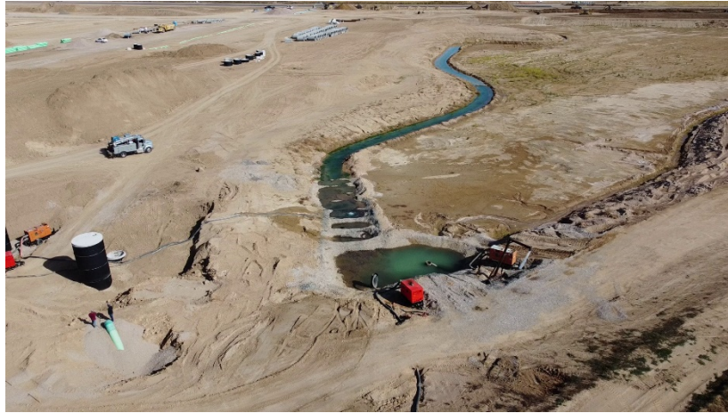
Prairie Song Pump House Location
